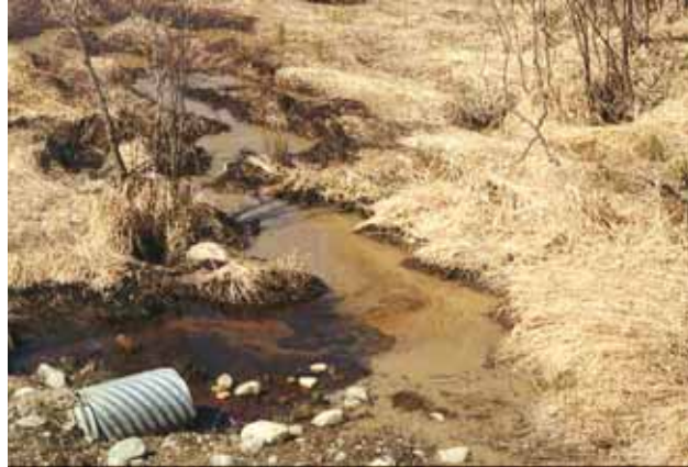
Figure 6. Sedimentation of stream from road runoff in the Houston Area.
