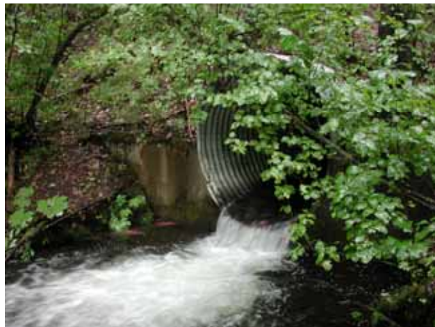
Figure 7. Perched outlet of the Question Creek culvert at the Talkeetna Spur Highway.
